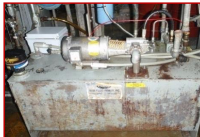
Fig 7: GPI CC Stack Reservoir
