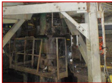
Fig 12: OCC Pulper Gearbox
